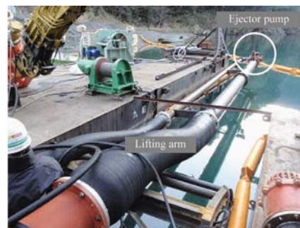
Figure 7. The photography of ejector pump and lifting arm.
