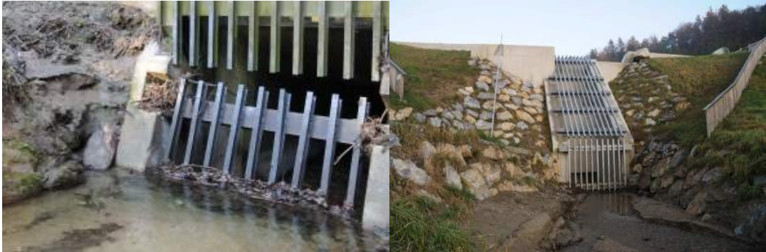
Figure 5: Screen bar design, and sediment and tree leaves trapping in front of a bottom outlet
