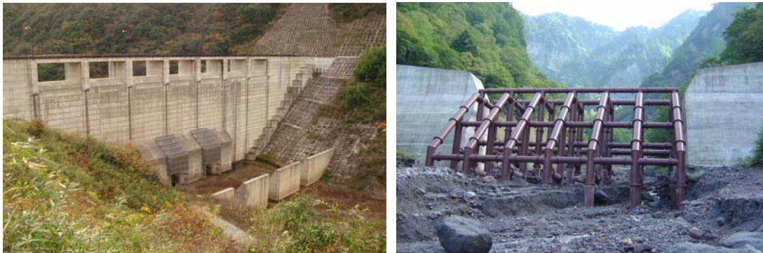
Figure 8: (left) Masudagawa flood mitigation dam; (right) Slit check dam from steel pipes
